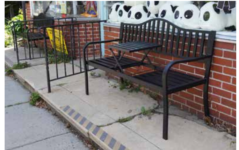
Unique benches with a pull-out tabletop are offered outside of this Main Street business, but the step is a barrier to accessibility.
