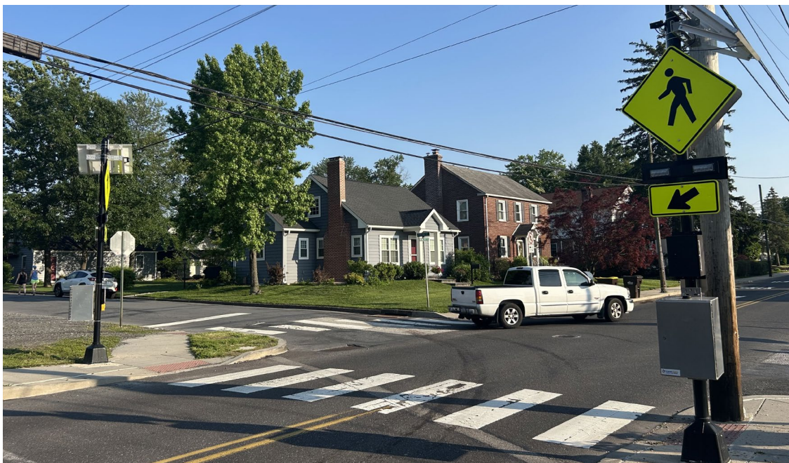
The new pedestrian-activated Rectangular Rapid Flashing Beacon (RRFB) enhances safety for those seeking to cross Walnut Street
